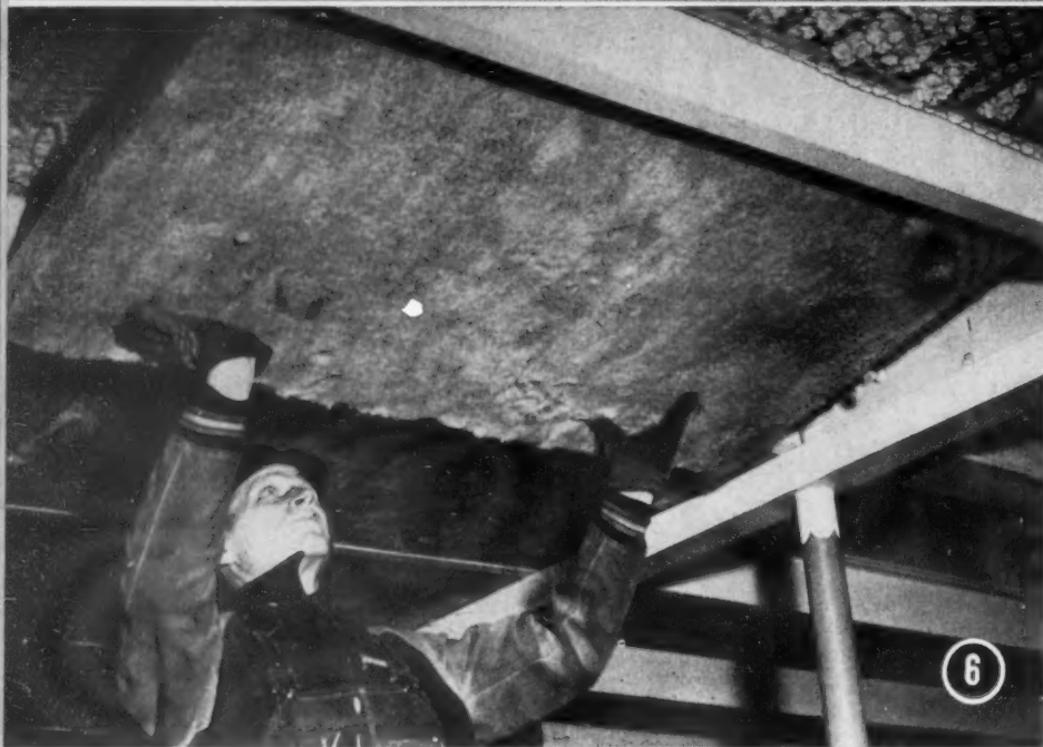
Fig. 6—Installing glass-fiber thermal insulation in the refrigerated compartment of a merchant ship
